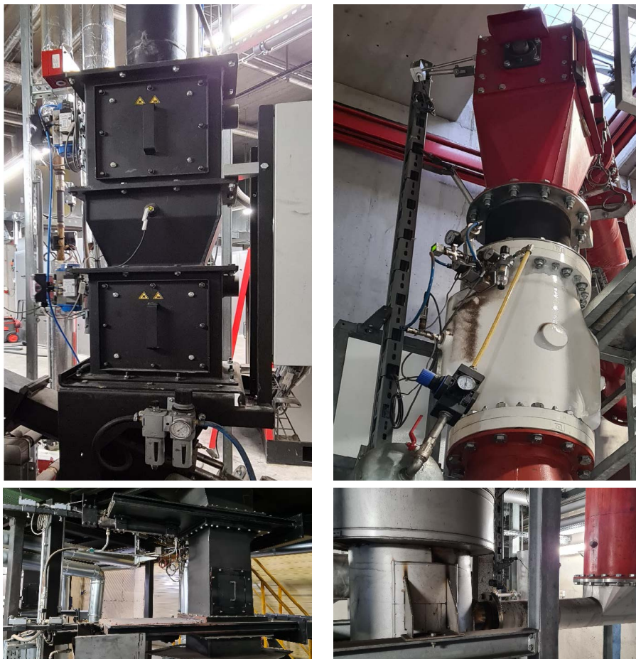
Picture 7: Safety devices upfront of the gasifier; top left: double valves; top right: combination of slider and air cushion; bottom left: double slider; bottom right auger screw into gasifier.
