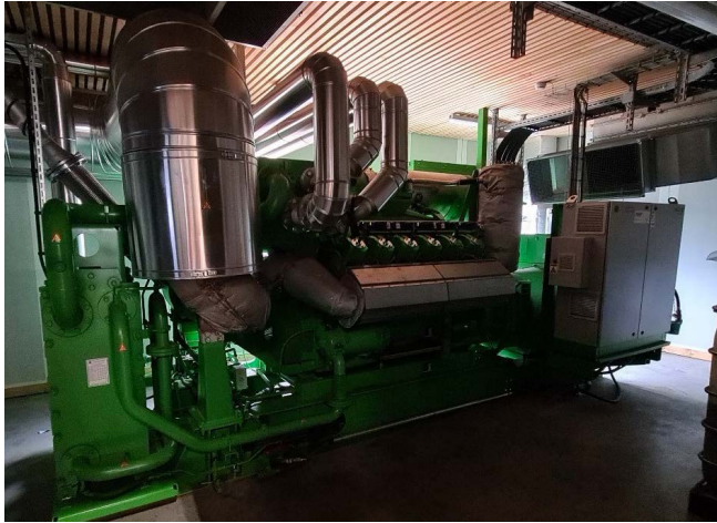
Picture 25: CHP unit to produce combined heat and power from wood gas.
