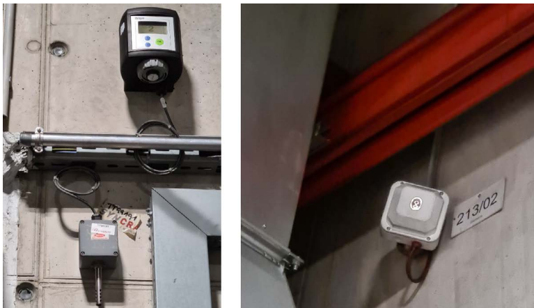
Picture 34: Fix installed safety devices (gas and flame detection).
