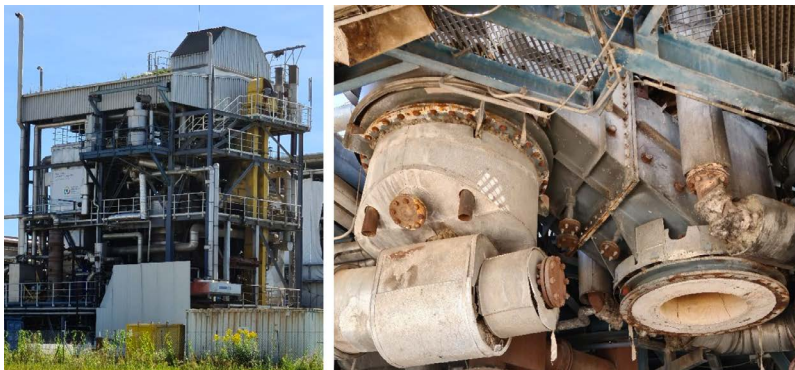
Picture 16: Fast Internally Circulating Fluidized Bed gasification plant in Güssing, Austria: left: whole plant; right: bottom of gasifier and autothermic bed recirculation chamber.
