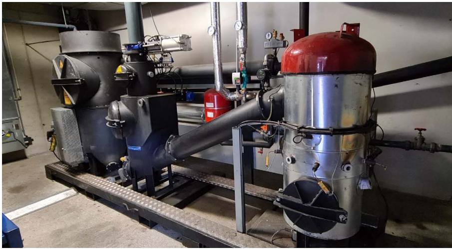
Picture 10: Downdraft gasifier with security system and feeding auger.
