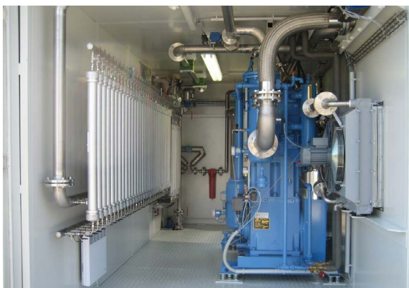
Picture 40: Piston compressor (right) with membrane upgrading system (left).
