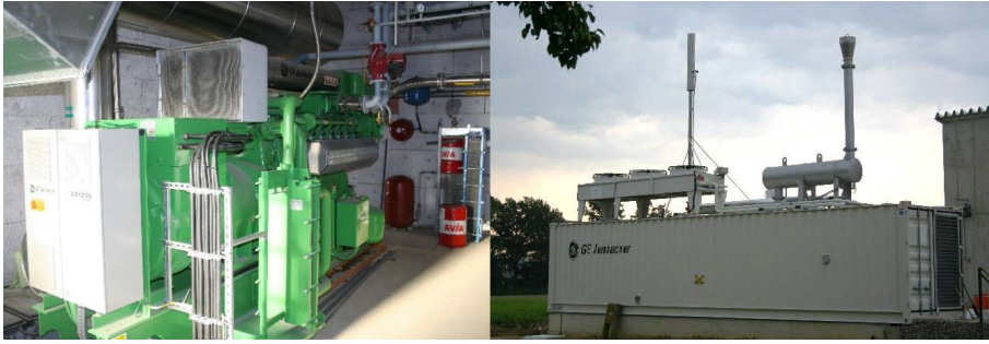
Picture 68: CHP unit: left: steered intake air, steering, generator, heat exchanger and gas engine, right: fully equipped CHP container with cooling, flare, heat exchanger and exhaust pipe above the container.
