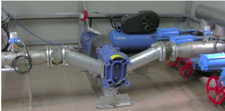
Picture 47: Pumping station with pressure sensor before and after the pump to detect distortions.
