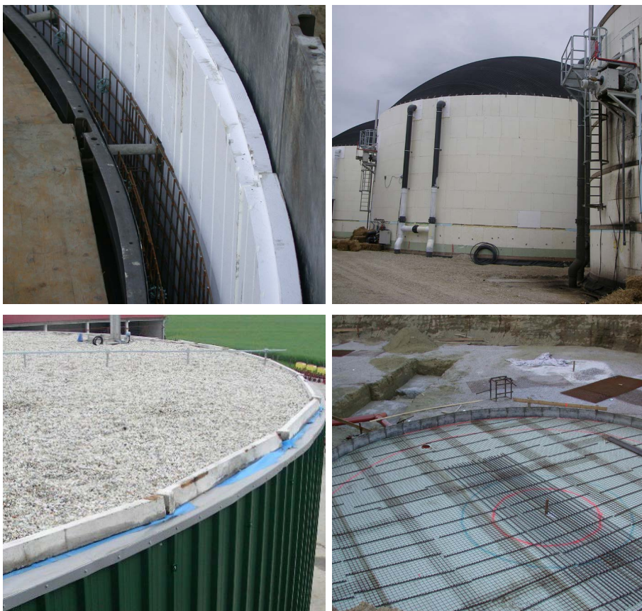
Picture 24: Types of wall isolation, top left: special confectioned isolation which is included in the process of casting the concrete, top right: isolation outside of digester through nails, bottom left: sandwich panels, bottom right: isolation under the floor.
