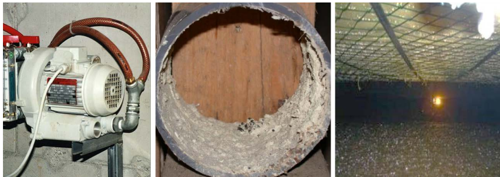
Picture 65: Left: blower for desulphuration with air, middle: elementary sulphur within a gas pipe, right: sulphur at the top of the digester.
