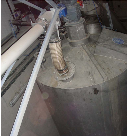
Picture 12: Substrate mixing tank followed by a feeding pump.
