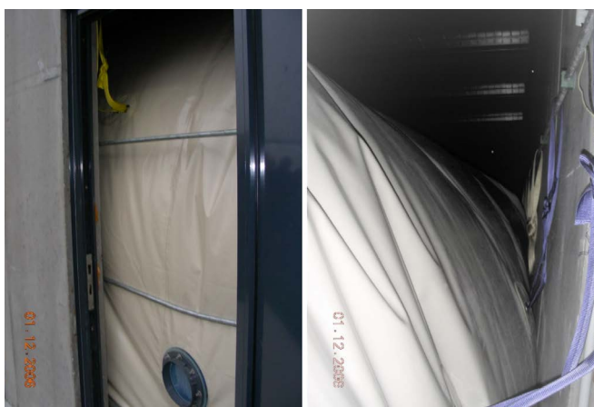
Picture 60: Single membrane gas storage in external housing.
