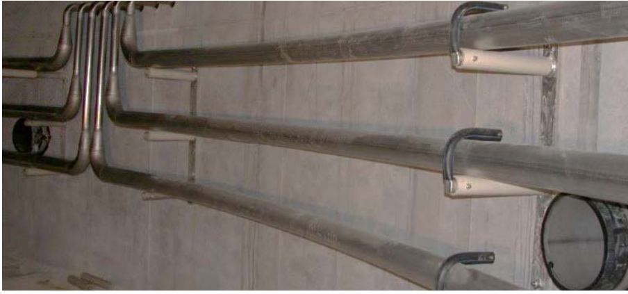
Picture 30: Stainless steel heat pipes directly attached to the digester wall. To avoid corrosion stainless steel pipes need to be installed galvanically isolated.
