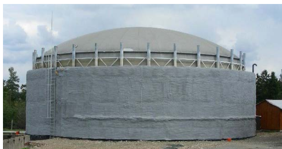
Picture 63: Wet gasometer directly included in the digestate storage tank.
