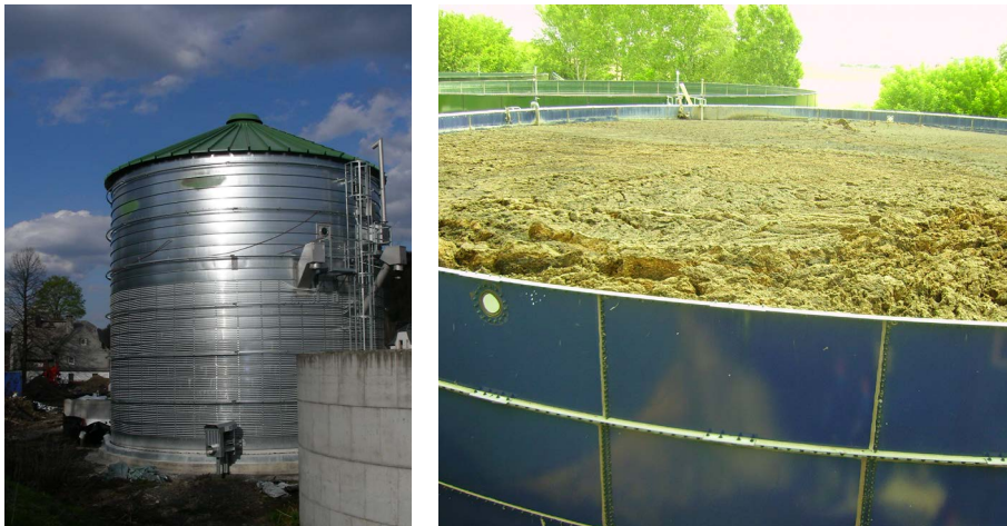
Picture 23: Digester material: left: rolled stainless steel digester with floor heating pipes on the outside, right: enameled steel storage.
