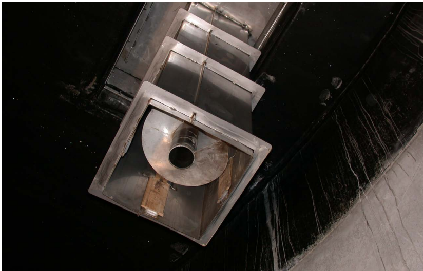
Picture 11: The feeding screw must always end below the liquid surface so that no biogas can escape.
