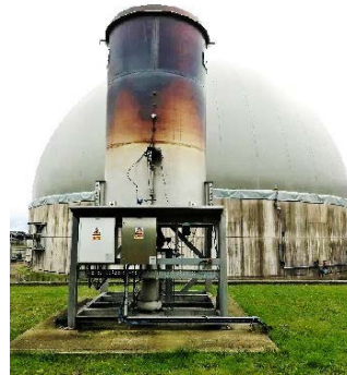
Picture 43: Enclosed flare in biogas plant.
