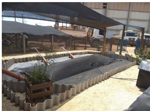
Picture 74: Plastic bag digester, Source: Ökobit.
