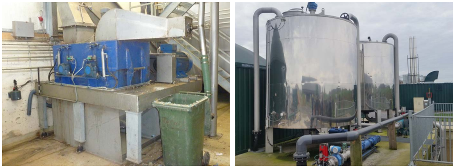
Picture 7: Left: unpacking machine for expired food with automatic separation of impurities, right: sanitation devices installed in parallel for higher performance.
