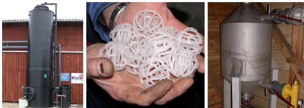
Picture 66: Left: external desulphurization column, middle: padding material for sulfobacter oxydans within external desulphurization column, right: activated coal filter.
