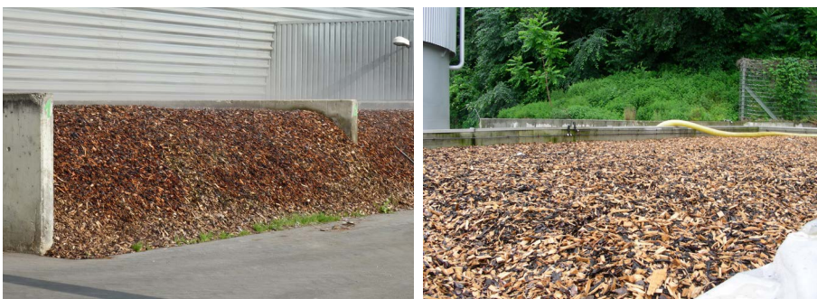
Picture 14: Biofilter filled with wood chip as bedding material for odour substance degrading bacteria.
