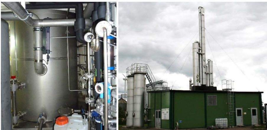
Picture 71: CO 2 separation through physical scrubber, left: scrubber column, right: physical scrubber installed in a container.
