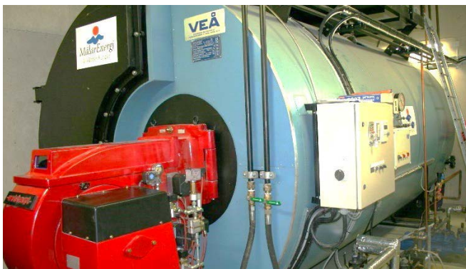
Picture 69: Typical peak load boiler for biogas with a capacity of 7.2 MW th .
