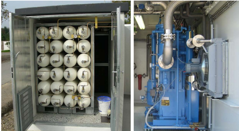
Picture 64: High pressure biogas storage systems with piston compressor.
