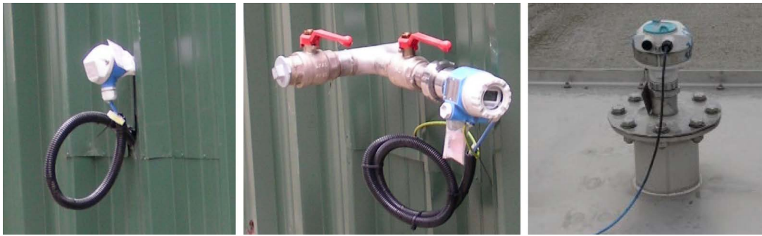
Picture 46: Measurement devices for temperature and level sensors (right: ultrasonic measures from top).
