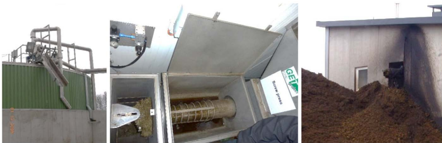
Picture 51: Screw press to dewater digestate.
