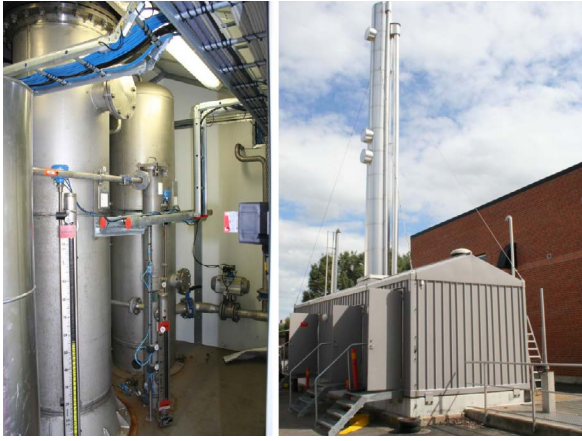
Picture 70: CO 2 separation through water scrubber left: scrubber column, right: water scrubber technique installed in a container.
