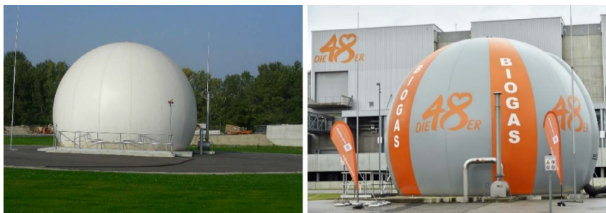
Picture 62: Stand-alone double membrane biogas storage systems shaped with air blower.
