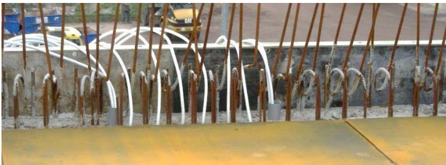
Picture 29: Heating system with floor heating pipes directly integrated into the concrete wall.
