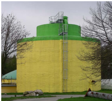
Picture 16: Hydraulic digester with the higher inner tank and the lower outer tank.
