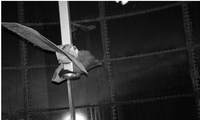
Picture 25: Vertically central positioned stirrer for a CSTR digester.
