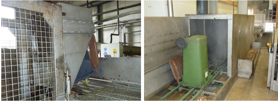
Picture 5: Top left: organic waste bin from catering and households, right: collecting lorry for catering and household waste with integrated emptying and cleaning device, bottom: organic waste bin emptying facility at the biogas plant with a subsequent washing-bay.
