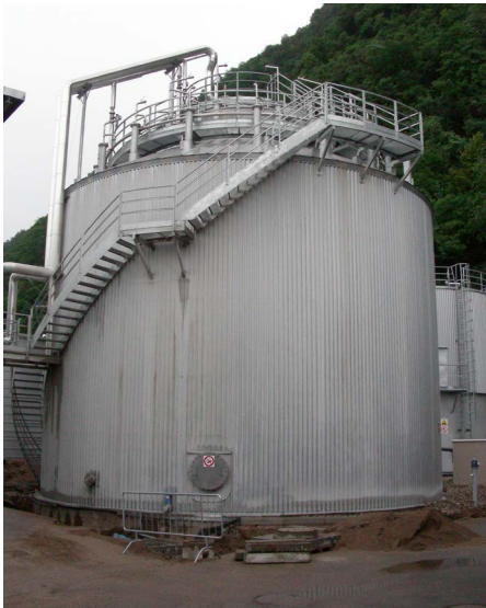
Picture 18: Upstream plug flow digester (UASB = up flow anaerobic sludge digester).
